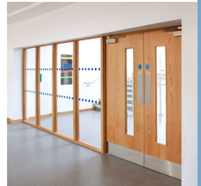
American white oak in a new academy in West Sussex. Where possible these doors are fitted alongside screens to allow for increased transition of light. These fire rated screens also create a feeling of openness and brightness conducive to a pleasant learning environment.
